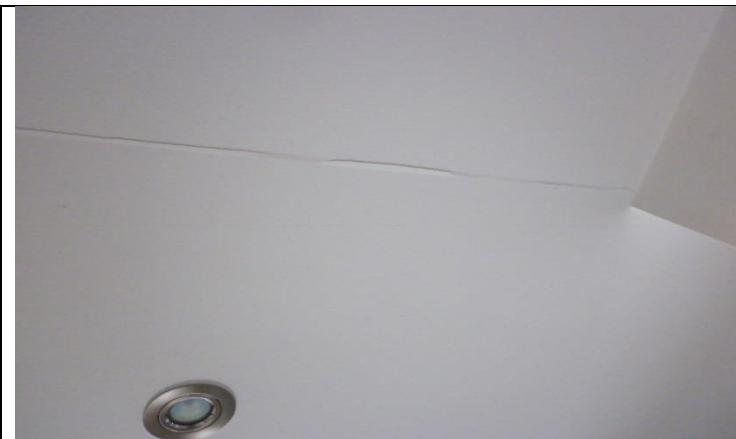
Crack in hall ceiling possibly due to it being a long hallway with no construction joint in the plasterboard. Suggest putting a construction joint in to stop future cracking.
