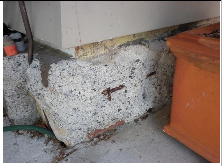
Exposed reinforcing in footing .Suggested plastering over footing to make good and keep steel from further rust.
