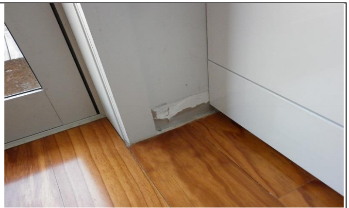
Skirting board missing in laundry.
