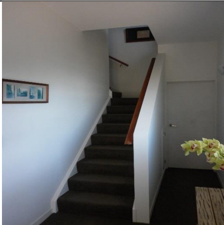
Stairs hand rail need to be repaired and fixings tightened or replaced.
